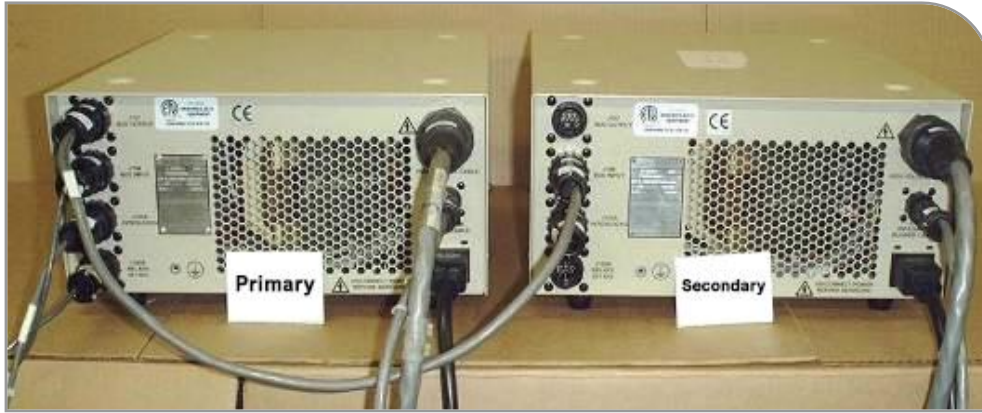
Figure 9. Power Supplies (Back)
